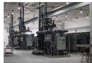
Carlton Treatment Plant
